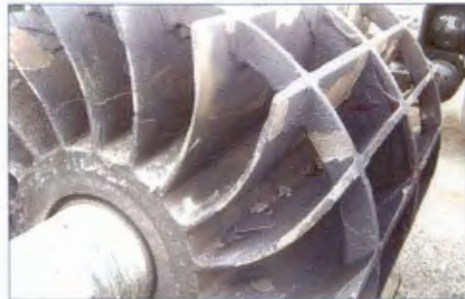
Damaged rotor before rebuilding
