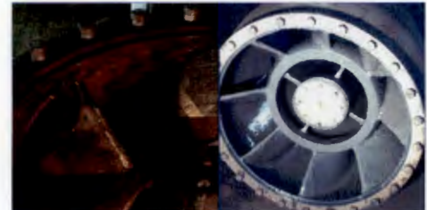
Diffuser vanes with steel gauze in place
